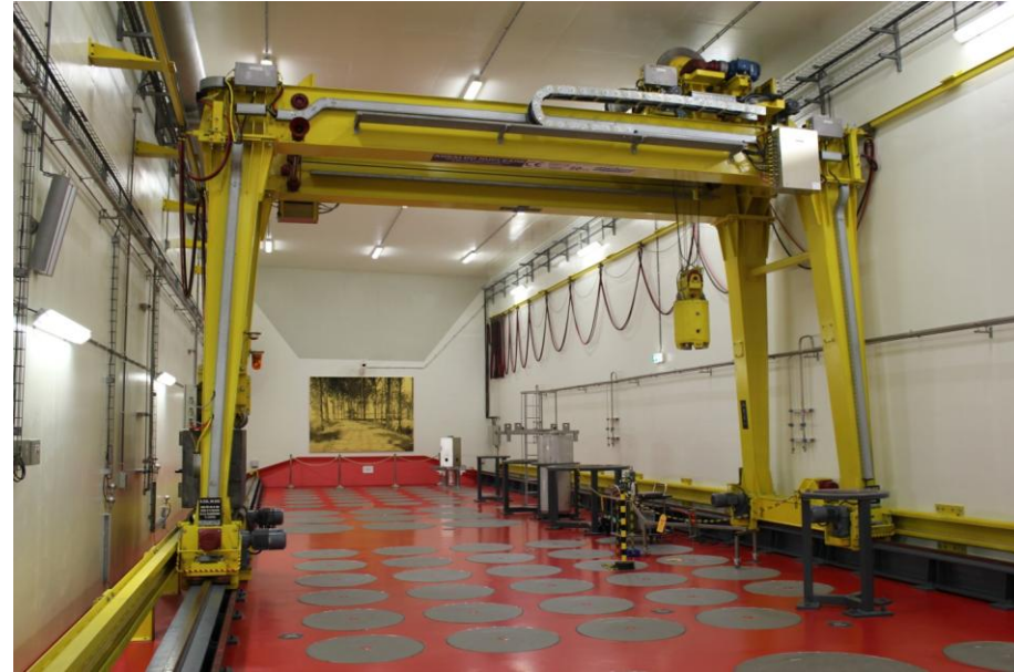
Storage module for heat-generating high level waste
