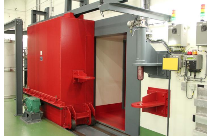
Heavy shielding door
